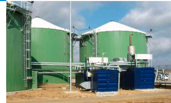
Biogas plant, Hostouň, Czech Republic
